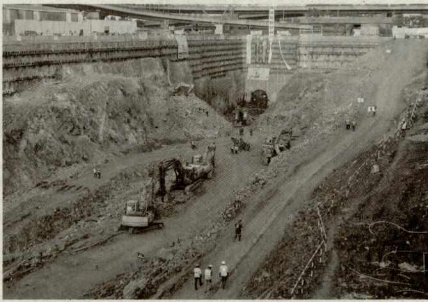
The TBM made the breakthrough near the metro construction site at T2 terminal of the Mumbai International Airport. —MRUGESH BANDIWADEKAR.
