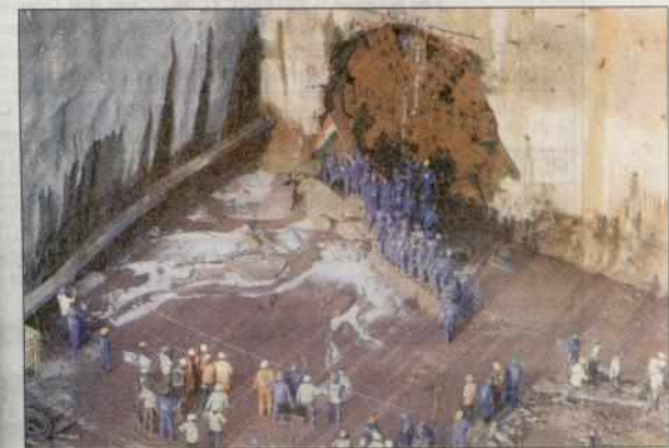
The first tunnel breakthrough of package 7 of the Mumbai Metro 3 was inaugurated on Monday. Dilip Kagda
