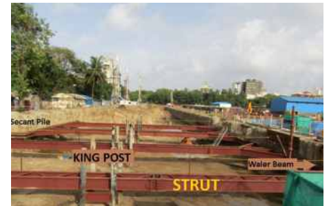
Supporting Members used in Deep Excavation of CST Metro station at the Azad Maidan (Mumbai)
