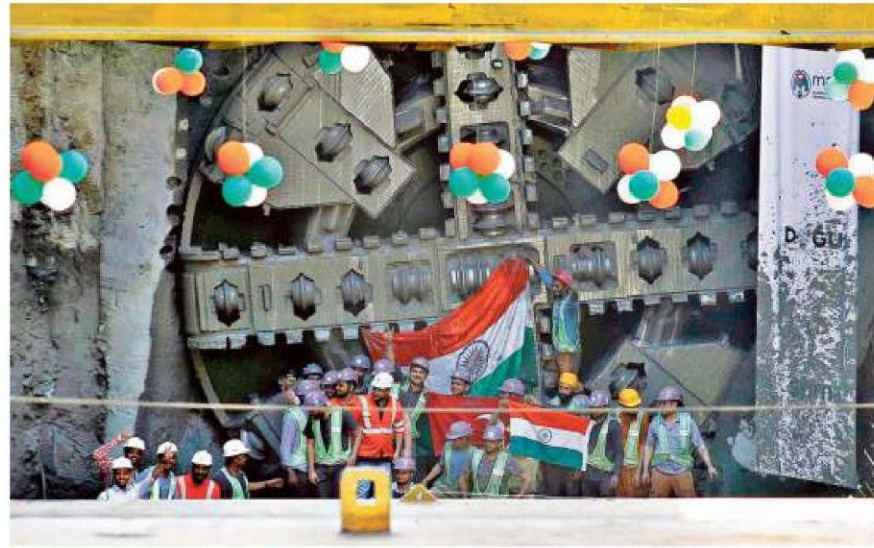
On track: Metro 3 achieved its 25th tunnelling breakthrough at Worli last week. ■ FILE PHOTO
