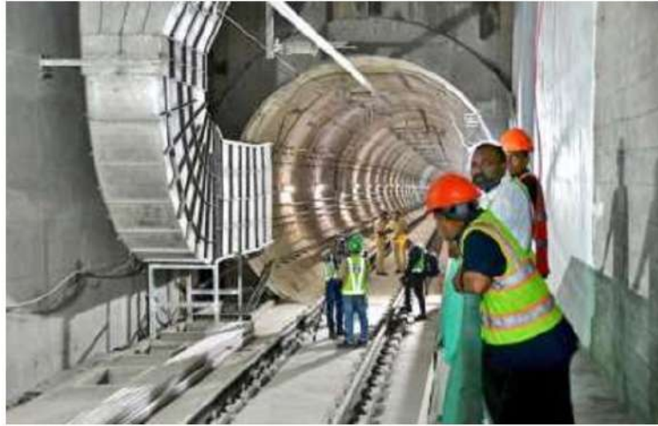
Construction work under way on the Metro Line 3 project at Vidhan Sabha Metro Station. FILE PHOTO
