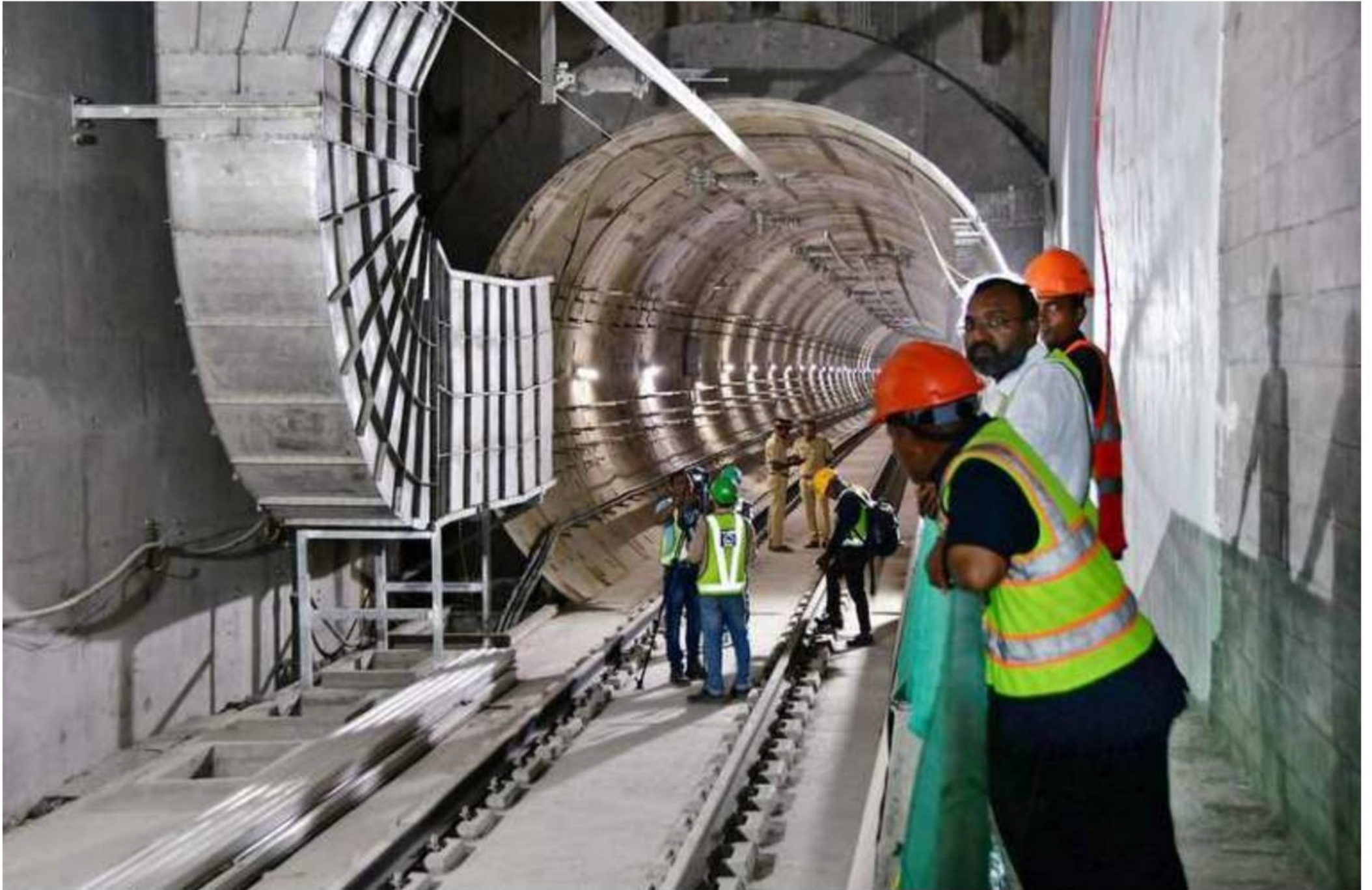
Construction work under way for Metro Route 3 project at Vidhan Bhavan Metro Station, Nariman Point, in Mumbai on Tuesday. PTI
